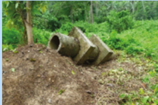
► Fig. 11. Hill collapsed on the Cabawan irrigation system's water impounding facility
