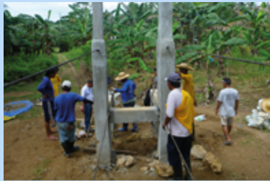
► Fig. 5. Workers replace the destroyed wooden footbridge with concrete and steel cable suspension bridge.
