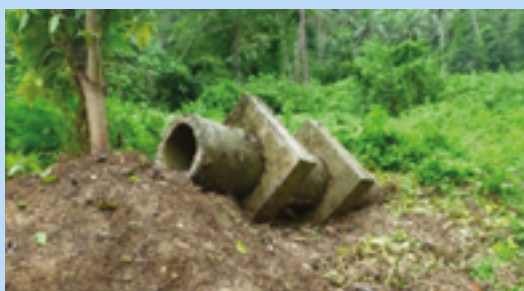
► Fig. 3. Damaged siphon stopped delivering irrigation water to the farmlands.
