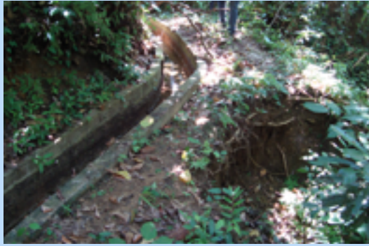
► Fig. 13. Collapsing ground underneath main canal.
