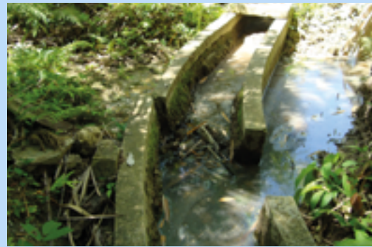
► Fig. 12. The earthquake damaged the irrigation system's main canal in several places
