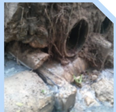
► Fig. 4. The earthquake broke the system's concrete pipes in several places, spilling precious irrigation water where it was not needed.
