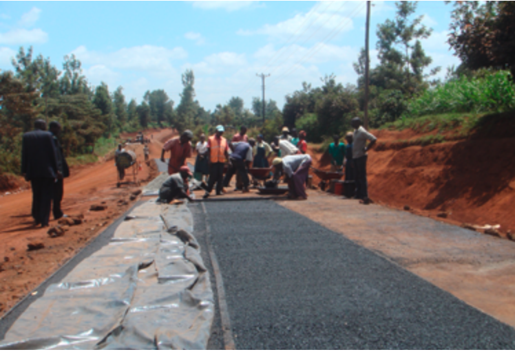
Sealing of a road using labour intensive methods under the Roads 2000 programme in Kenya (Credit: ILO)
