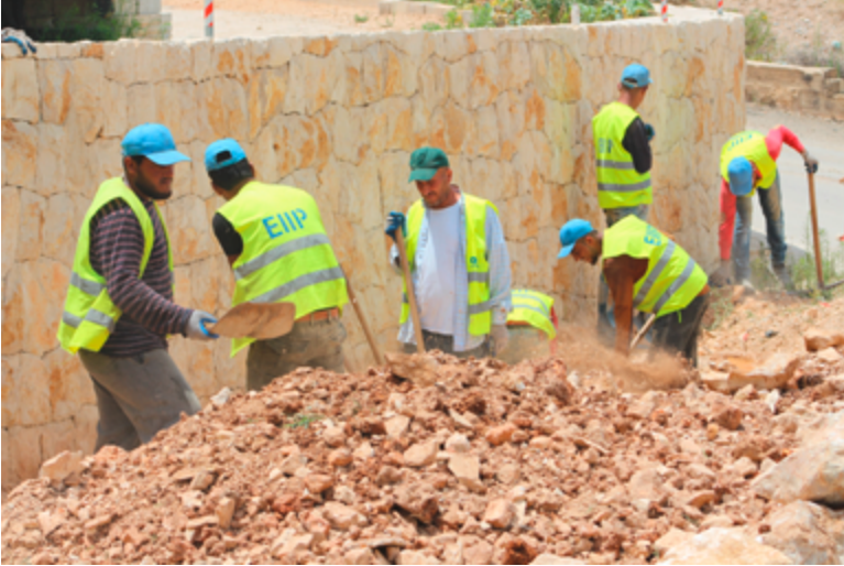
Workers building storm water drains in the town of Mazboud in the Chouf district in the Mount Lebanon area, under the Employment Intensive Infrastructure Programme in Lebanon (EIIP) (Credit: ILO)
