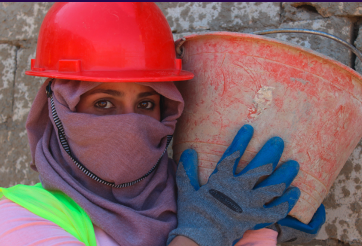
Working on a water reservoir to serve the town of Hamanna to the east of Beirut in Lebanon, under the Employment Intensive Infrastructure Programme in Lebanon (Credit: ILO)
