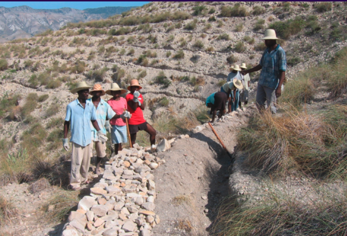
Construction of contour ditches to reduce erosion and runoff in Gonaives, Haiti as part of rehabilitation works after hurricane Jeanne, 2005 (Credit: ILO)
