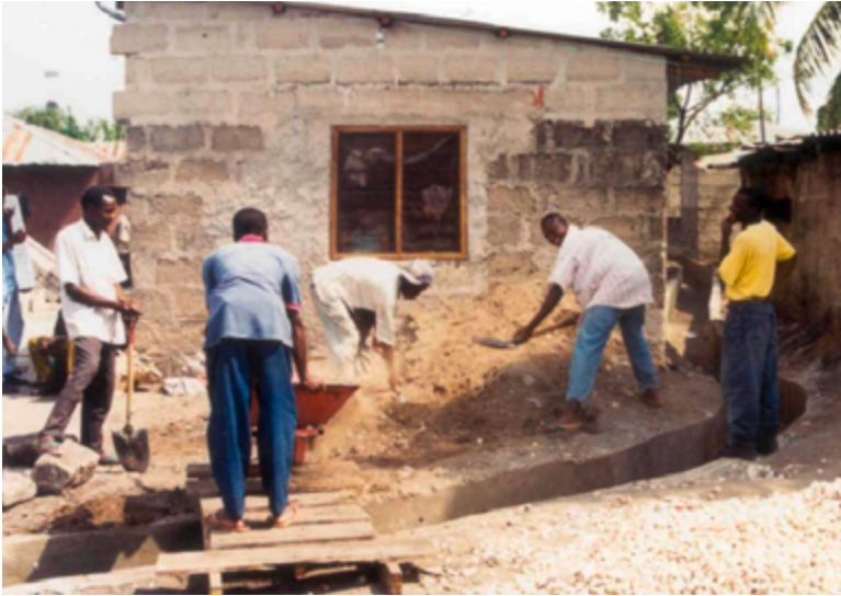
Construction of urban drainage works as part of the Hanna Nassif Community Upgrading Project in Dar es Salaam, Tanzania, late 1990s (Credit: Unknown)
