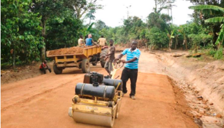
Compaction of a gravel road using a pedestrian roller in Ghana (Credit: Htun Hlaing)
