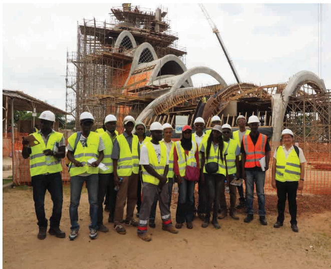
CNP WISCON trainers conduct visit to a construction site with work at height. Nianing, July 2017.
