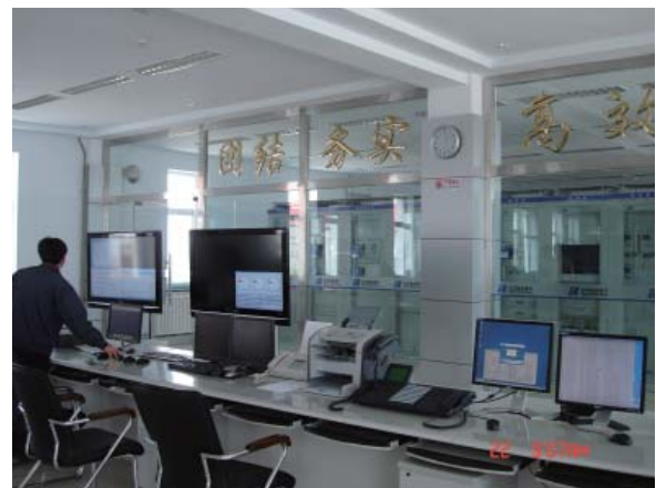
A central control room of the thermal power plant
