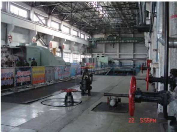
Boiler workshop of the thermal power plant
