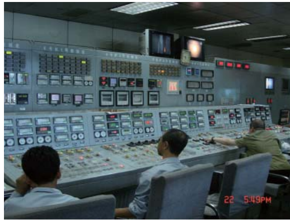
A central control room of 10,000 KW thermal power plant
